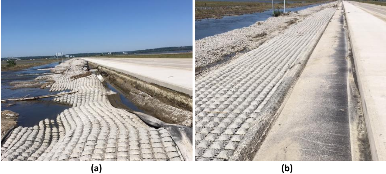
Figure 5. (a) Failed Grid Matting and (b) Asphalt Wedge Placed to Assist in Maintaining Mat Stability (Photo Credit Dr. Scott Schram, Iowa DOT)
