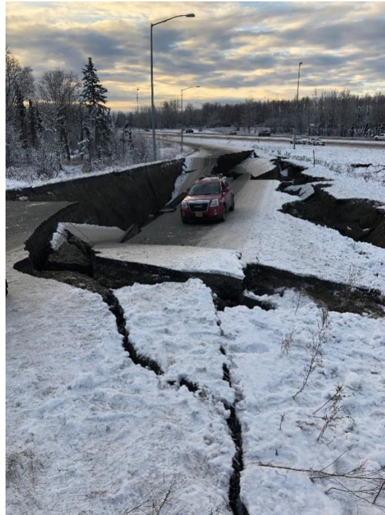
Figure 7. Failed Section of Minnesota Drive Ramp after 2018 7.0 Alaska Earthquake ( Photo Credit Knik Construction )
