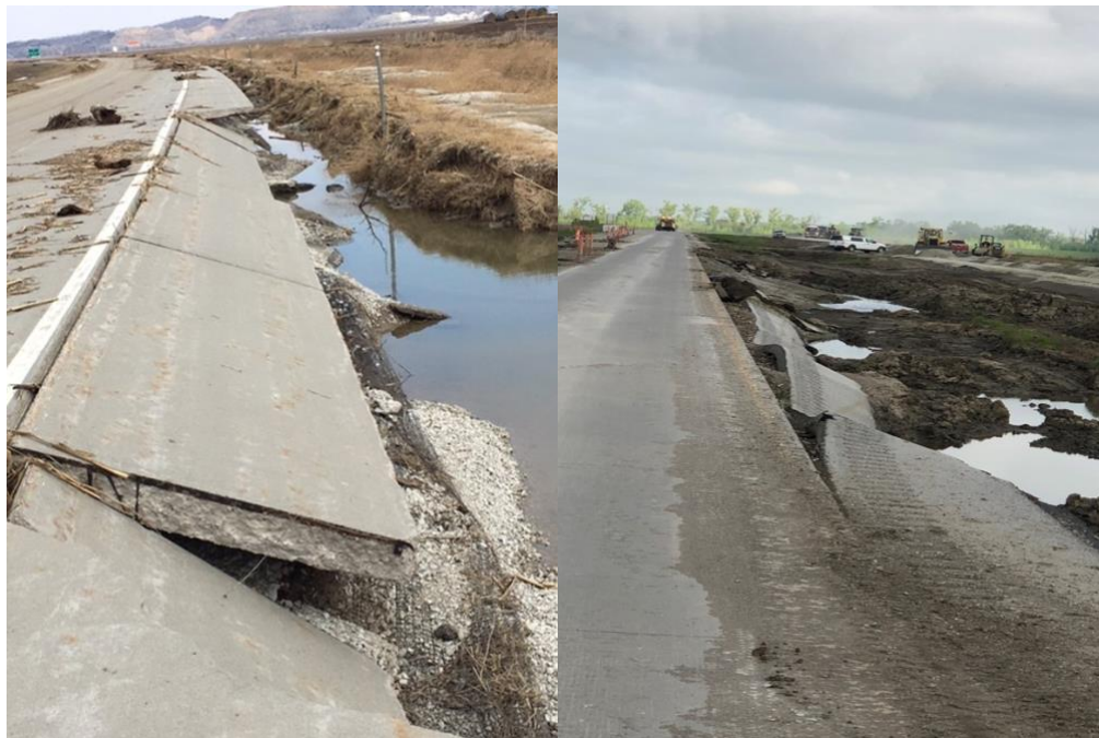
Figure 3. Shoulder Failures as a Result of Flood Water Undermining (Photo Credit Dr. Scott Schram, Iowa DOT)
