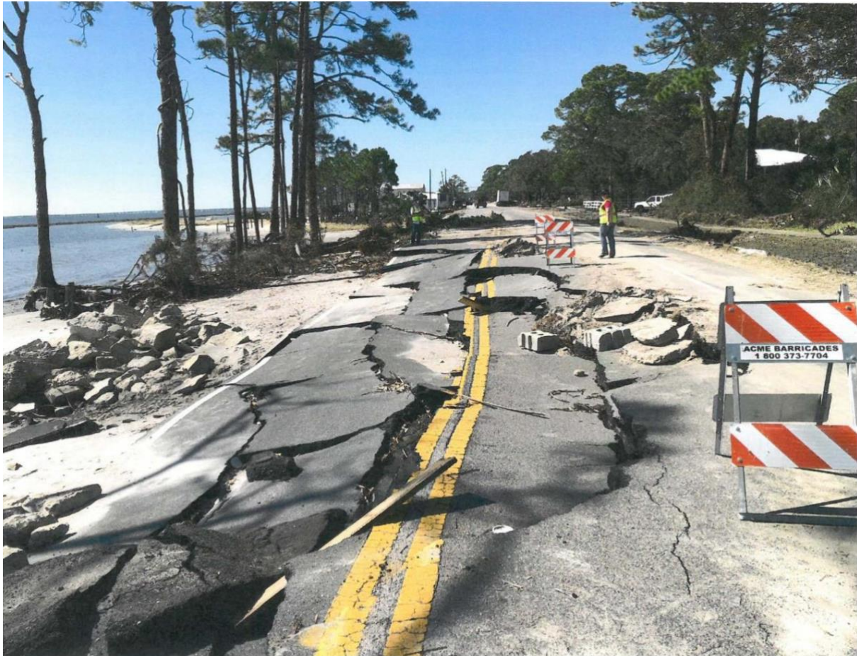
FIGURE A1. Hurricane Damage as A Result of Hurricane Michael on State Route 30 (US-98) in Franklin County Florida (Photo Credit Kevin Wall, Anderson Columbia)
