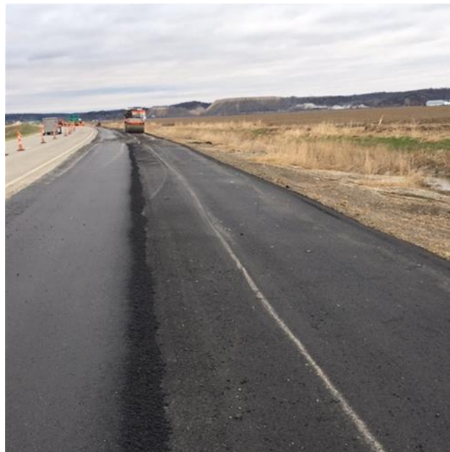
Figure 6. Extended (Additional) Shoulder as Temporary Flood Mitigation Technique in Case Additional Flooding Occurred Before Geogrid Mats Were Installed
